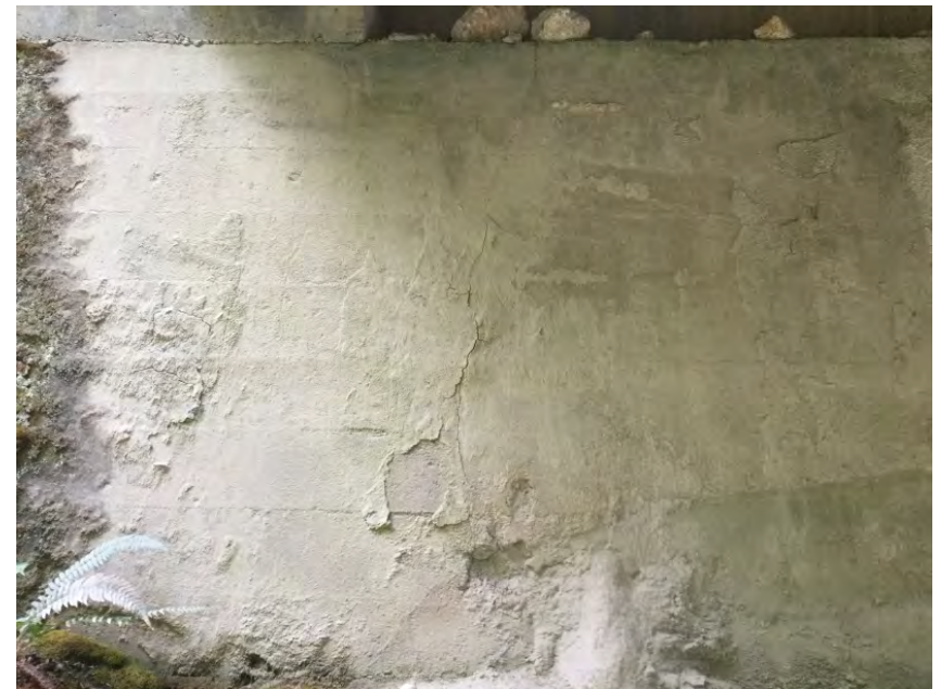
Vertical crack in CIP, under upstream girder left bank
