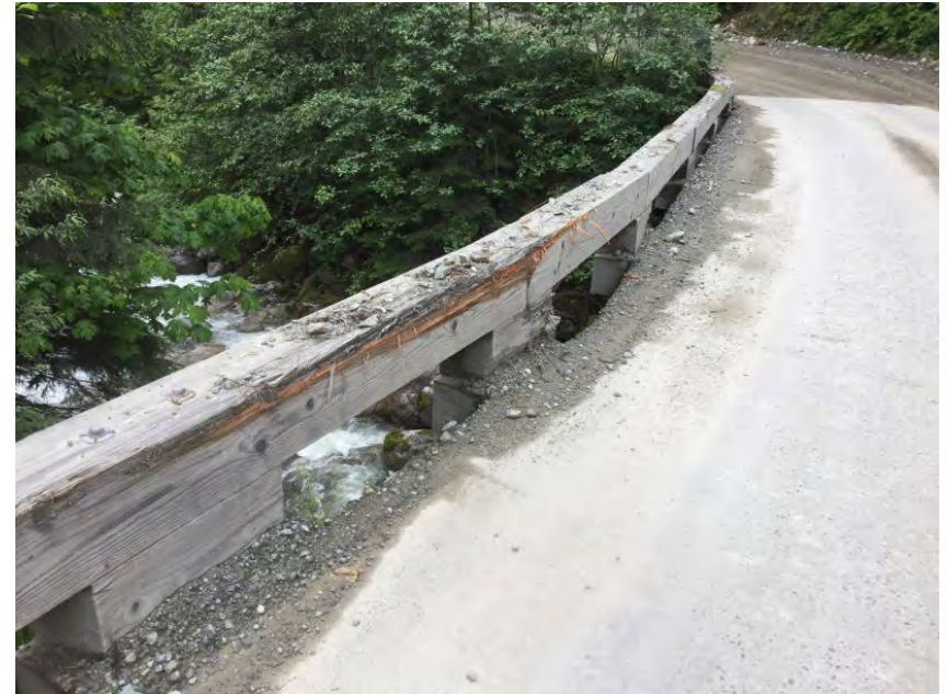
Recent damage to rail but still functional
