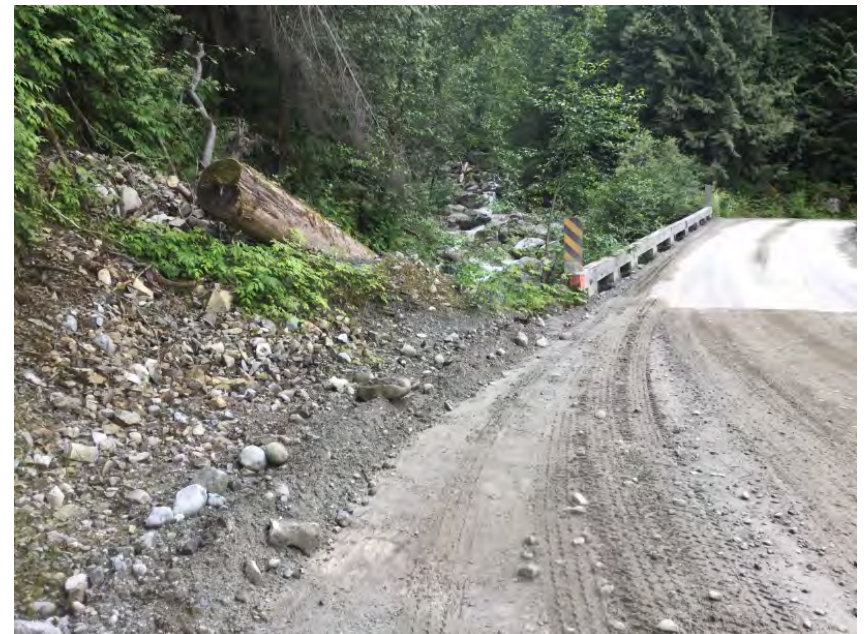
Missing fender at upstream right approach
