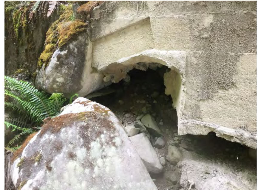
Hole in bottom of CIP, right under girder (upstream left bank)
